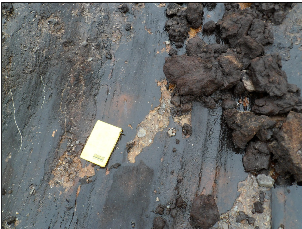
Figure 4.5: Base of Peat failure, Flughland, Co. Donegal, 2017. (Photo courtesy of Dr Paul Jennings)
