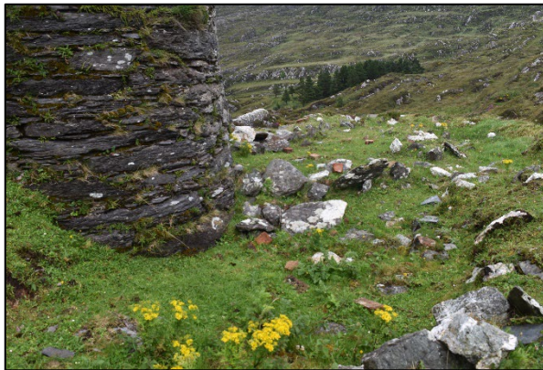
Base of Coom engine house chimney, showing accumulation of bricks that have fallen from chimney.
