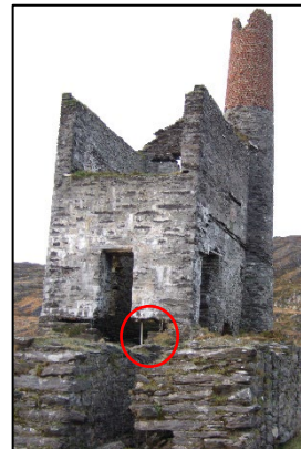
Coom engine house in 2008 – note greater height of chimney compared to recent photo (above). Steel support apparent in 2008 (red circle) now absent.
