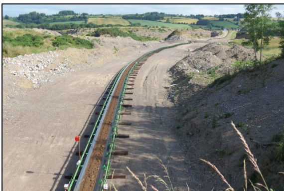
Sand and gravel conveyor crosses under the road at Garryhesta. Looking north.
