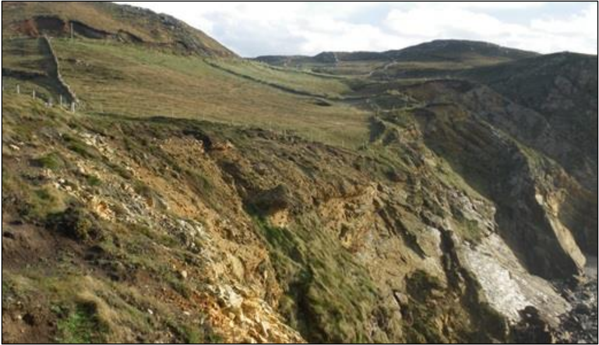
Crohy Head site: general view from north with cliff excavation in foreground.
