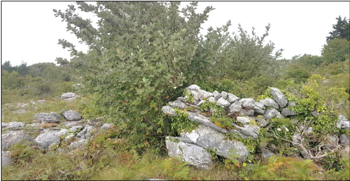
Mushroom rock – part of a drystone wall, partially overgrown by ivy and tree cover.
