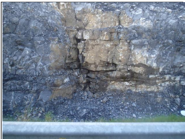
Cavity in karstified bedrock along the eastern side of the cutting.
