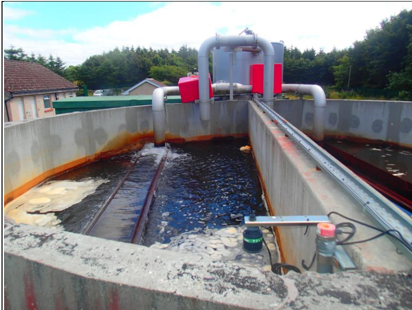
One of the water treatment tanks within the spring compound, July 2018.
