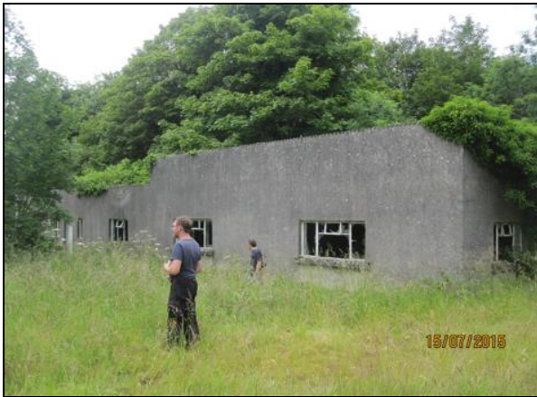
The former Administration Block is now derelict.
