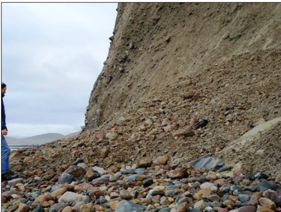
Deposits of mud, sand, gravel, cobble and boulders after a cliff face collapse.
