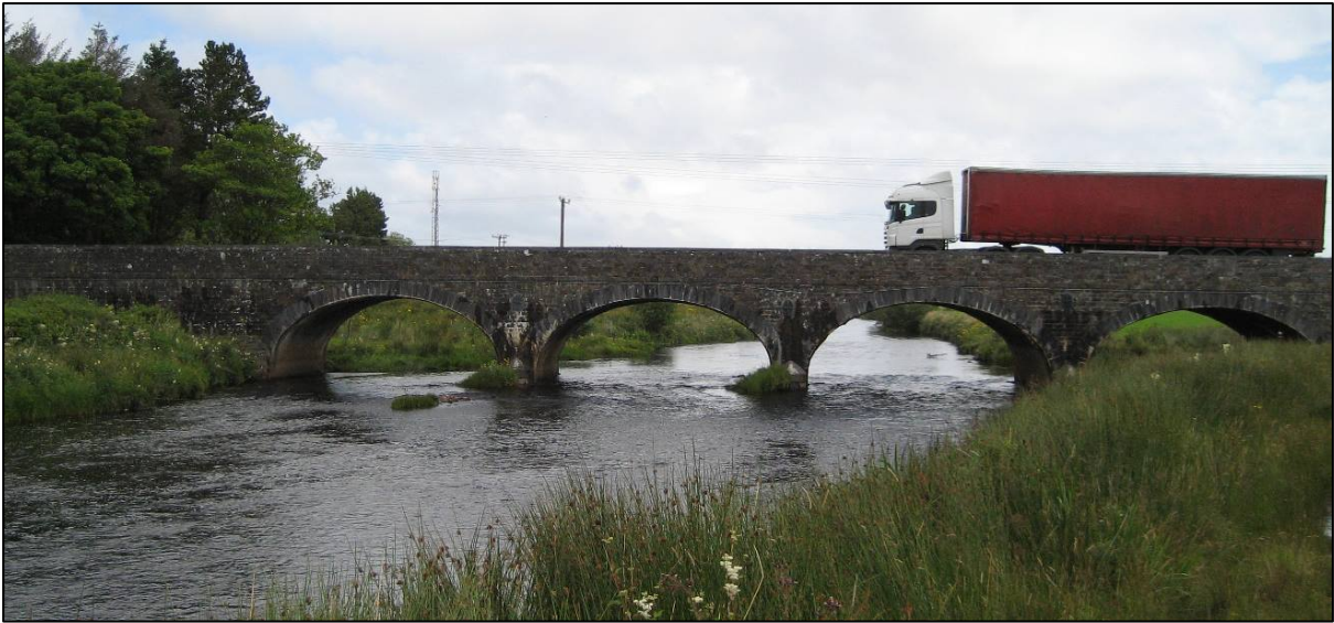
Bellacorick Bridge ( Musical Bridge ) viewed from the south looking upstream to the Oweninny River.
