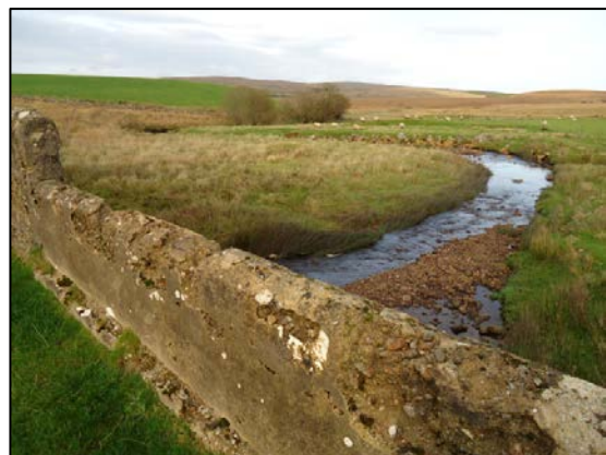
Derrycraff River viewed from low bridge at Derrycraff, looking NE. The riverbed is predominantly loose gravel and cobbles. No bedrock can be observed in the river bed for c. 500m downstream from bridge.
