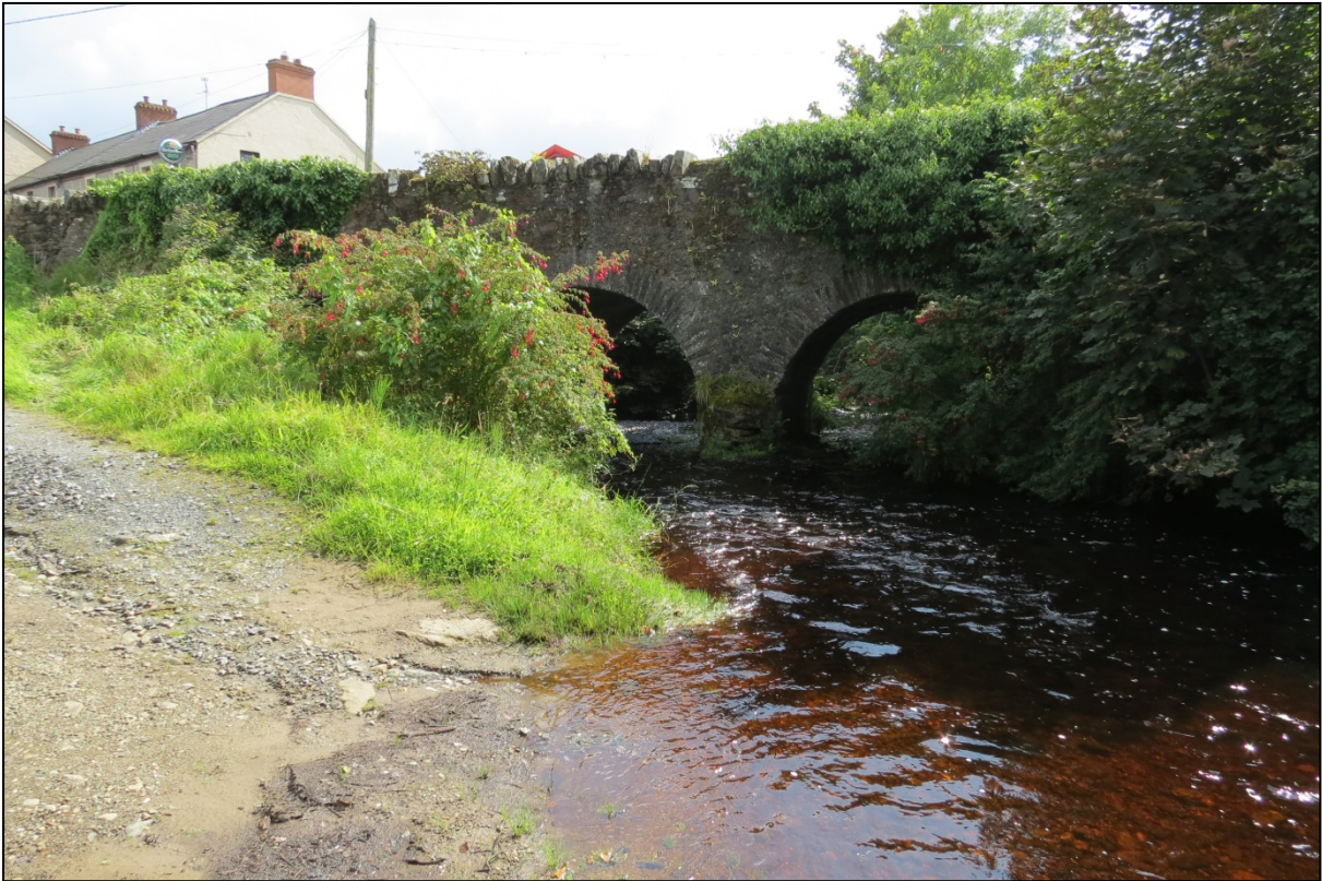
Cabry River - view downstream (southeast) at three-arch stone road bridge at Carrowkeel.
