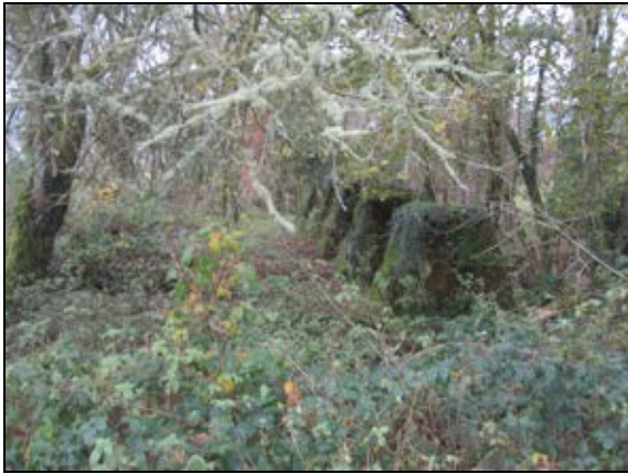
Concrete pillars that once supported some process on site, possibly a small railway.
