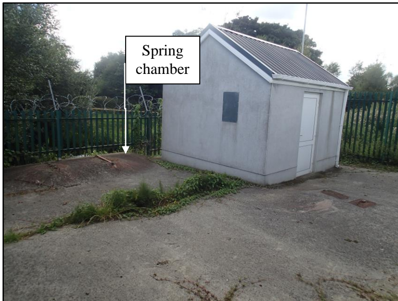
The pumphouse compound with the spring completely encased within the subsurface chamber.
