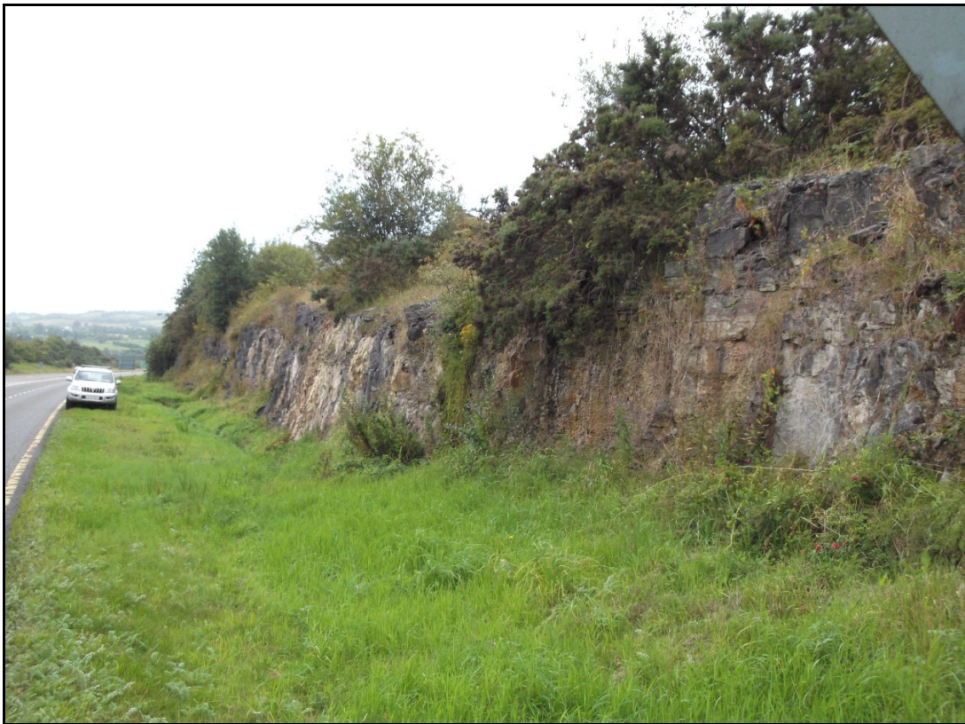
The mid-section of the Boyle Road Cutting showing the wide verge and relatively unvegetated cliff.
