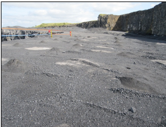
A bench that has been drilled ready to place explosives in the pattern of holes to blast the rock apart in a highly controlled operation.
