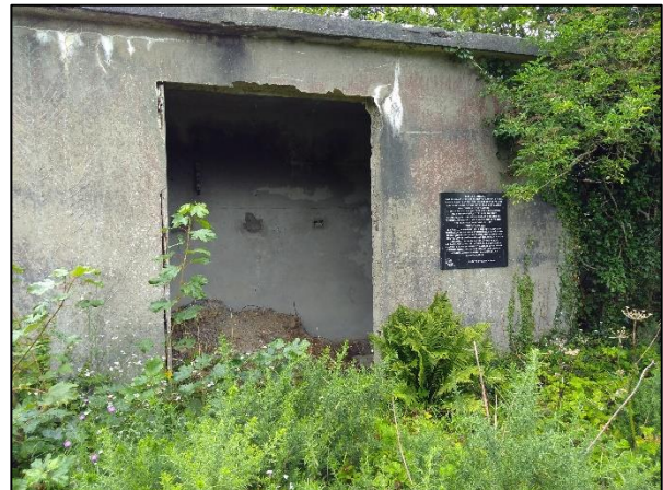
Remains of pilot Waelz processing plant (1950) built to recycle zinc left in slag heaps after 19 th century mining at Ballygown.
