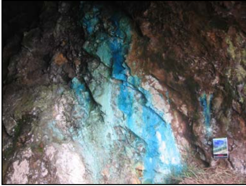
Blue copper gels stain the walls of some of the adits but they are wet and easily damaged.
