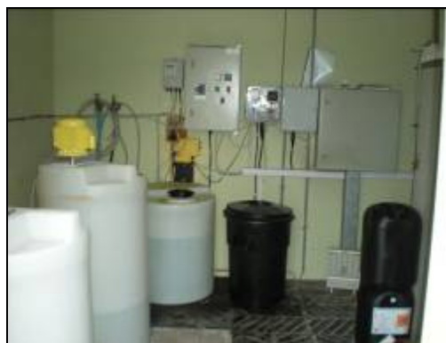
Photo 6: Chlorine Treatment in the Pump House
