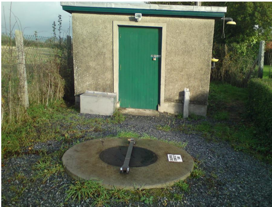
Photograph 1 Borehole housing and treatment works
