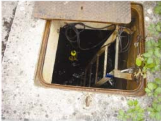
Photo 2: Holding tank and Aquasil feed
